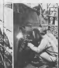
ARUBA ORANJESTAD as machinist. A welder works on her (two photos). Completing the Oranjestad as she ditches. She was scheduled
